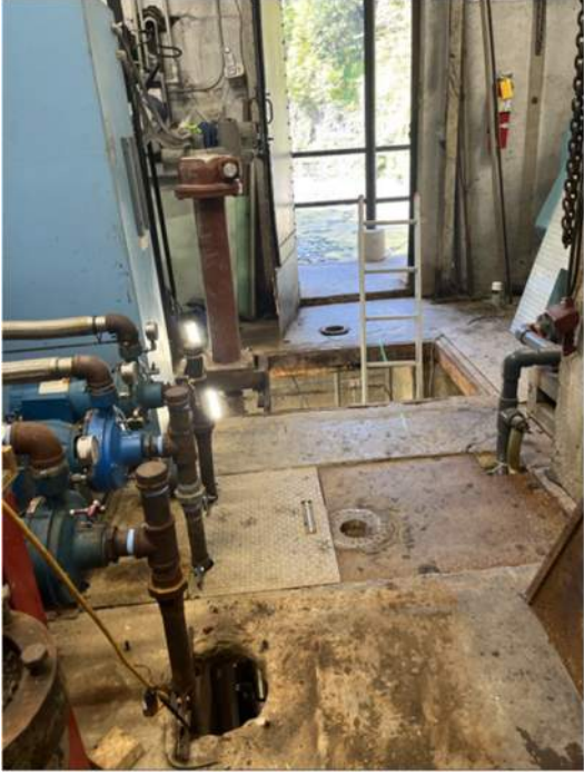
9/28/2023 – looking into first opening just inside the door of the gatehouse. This is middle chamber of the lower level.
