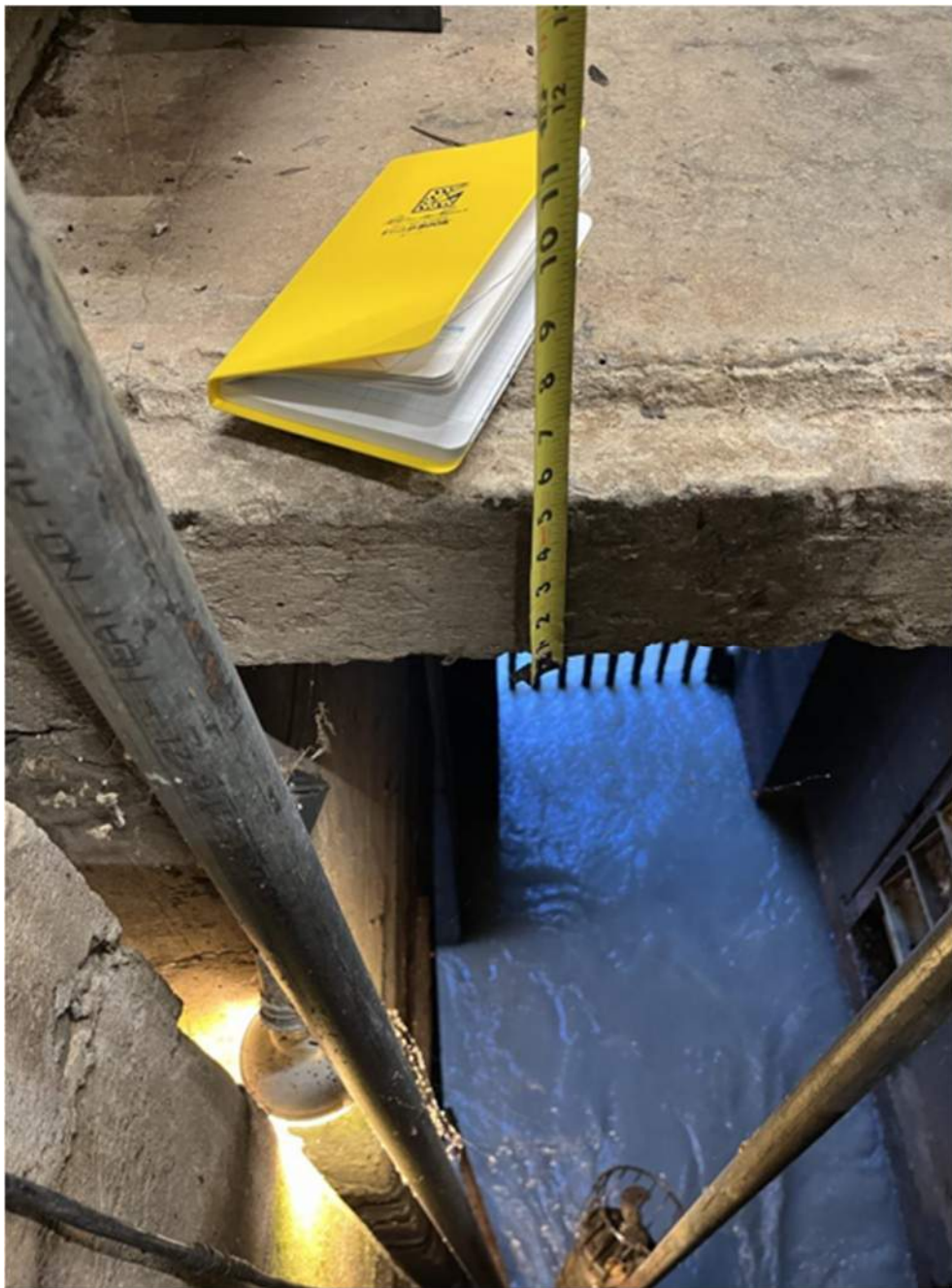
9/28/2023 – looking into lower level of the gatehouse at intake trash rack. This is the first chamber of the lower level.
